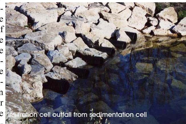
Back-pitched pipes from sedimentation cell to infiltration cell
